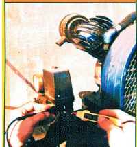
TESTS DC VOLTAGE
